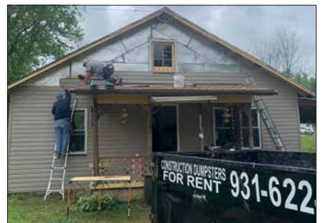
SIDING - A duo of volunteers, one a long-time engineer and the other a lawyer, add siding to the second story of a Fairgrounds Dr. home.
